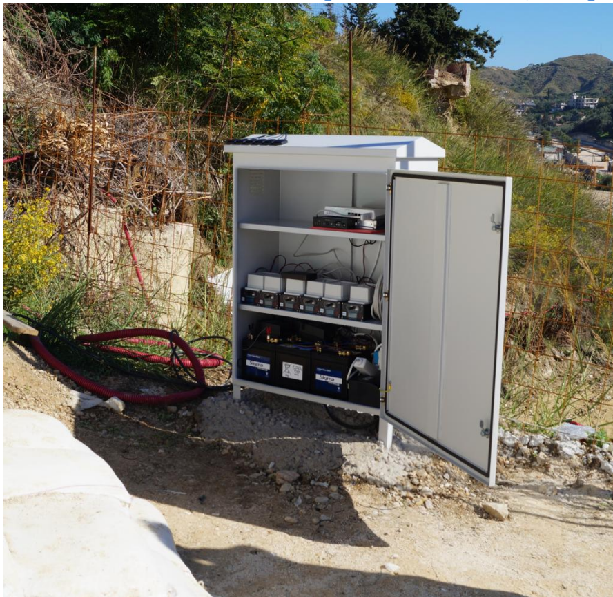
Figure 9: Monitoring System shelter.
